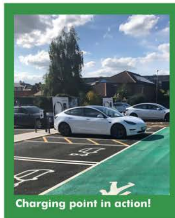
The installed charging point
