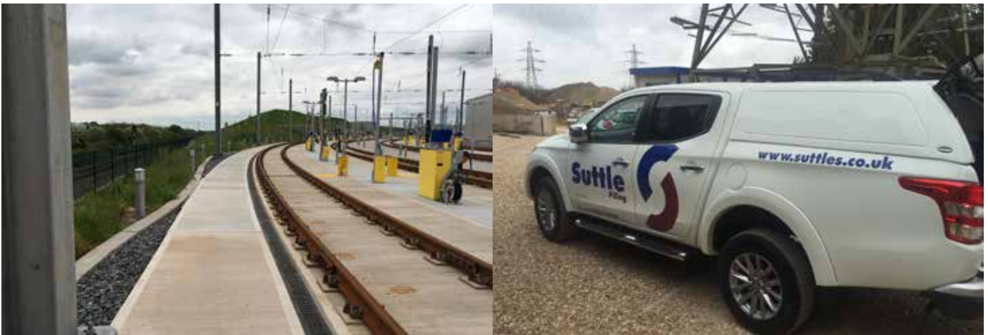
New contracts: (l-r) the line at Stoke Gifford, and the newly branded Suttles Piling pick-up
