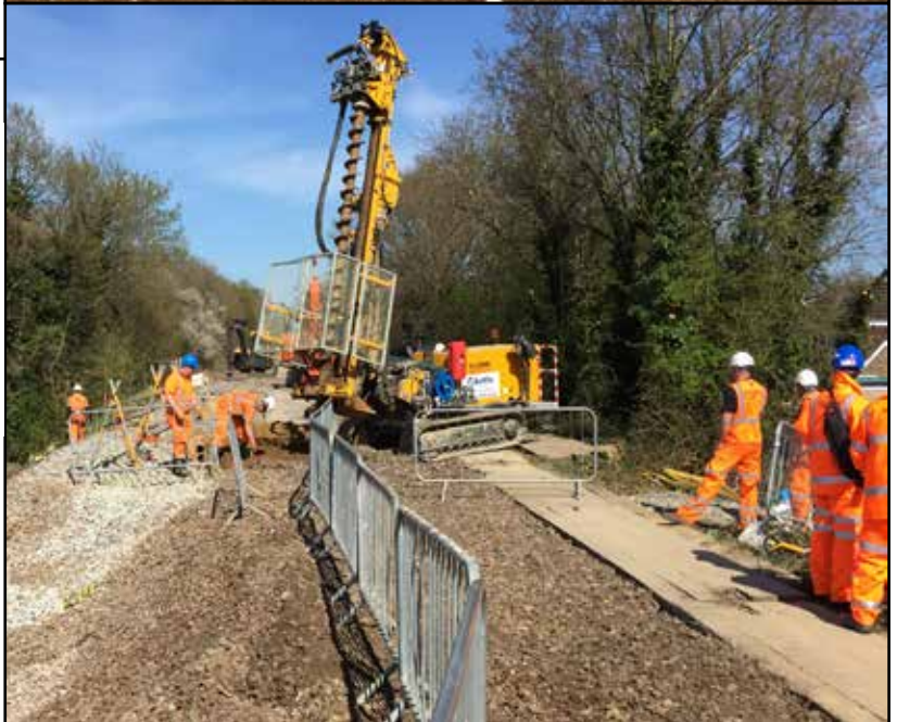
Ahead of schedule: a failed railway embankment between Farnham and Alton required pre-drilling and sheet piles
