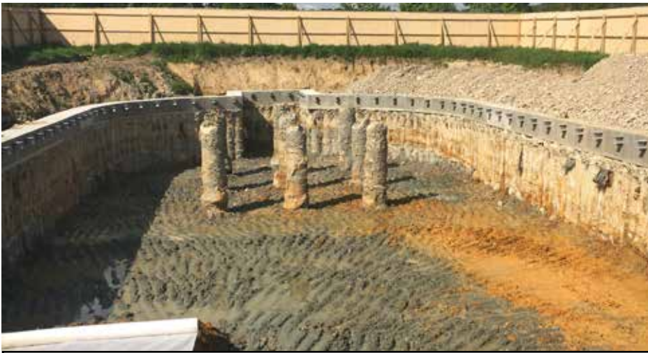
Breaking new ground: the secant piling at Woodlands Burial Ground was a first for Suttles
