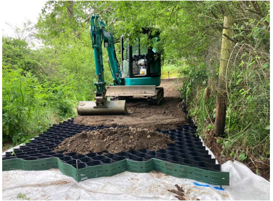
Figure 3: The recycled Type 1 sub base being used to infill the cellweb base product that is under the pathways.
