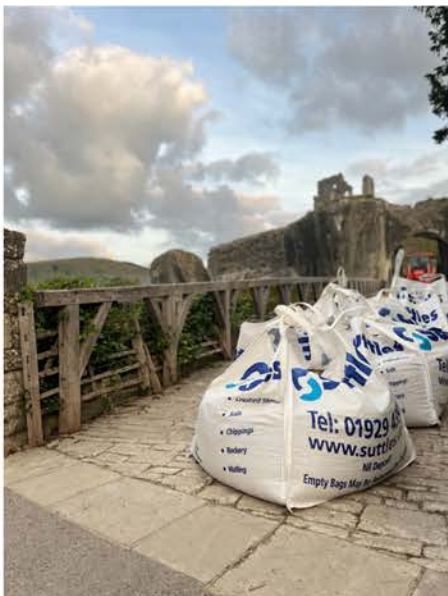
Figure 4: The bags on the bridge having been unloaded from the HIAB and waiting for the tractor.
